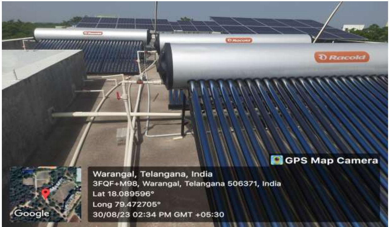
Solar water heater
