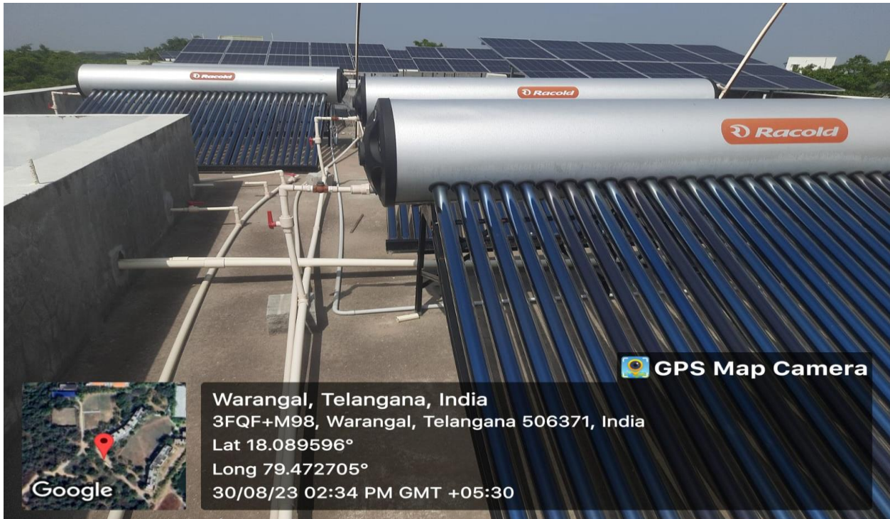
Solar water heater
