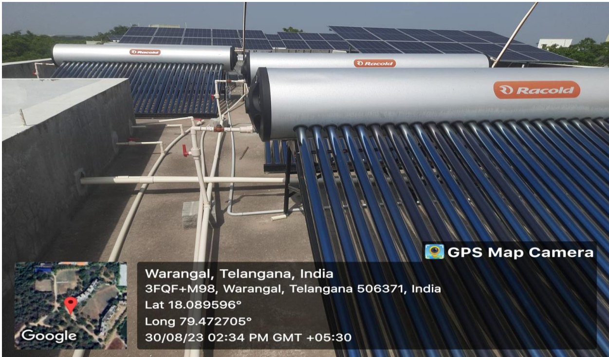
Fig: Solar water heating system
