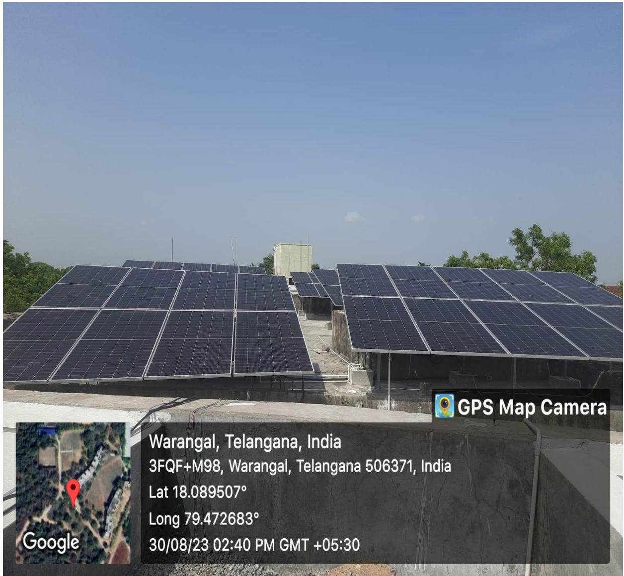
Fig: Solar power panel
